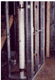
The GFX S3-60 serving two bathrooms in typical house
