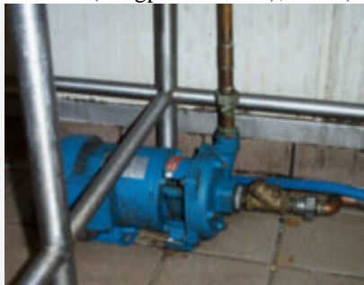
(e) Variable speed wastewater pump
