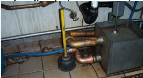
(f) Wastewater holding tank with automatic bypass
