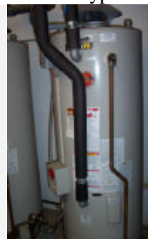
(g) One of three A.O. Smith MasterFit® induced draft tank-type commercial gas water heaters (Model BTR 500)
