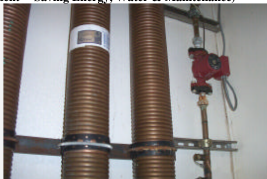
(b) Three speed Grundfos UP15-42F Circulator (Circulates cold & preheated water between 4 GFX-coils & 3 85-gallon gas water heaters @ 4.7, 5.8 or 6.5 gpm)
